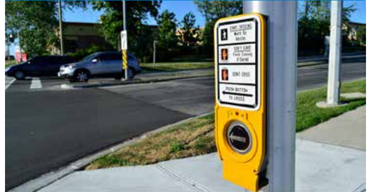
Upgraded Push Buttons / LPI
