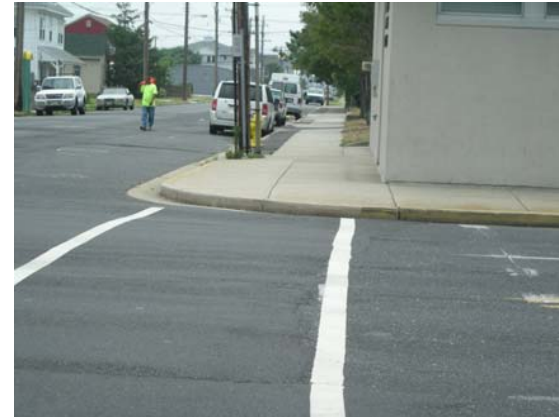
PICTURE 2: NO CURB RAMP AT CROSSWALK AT GARFIELD AVENUE
