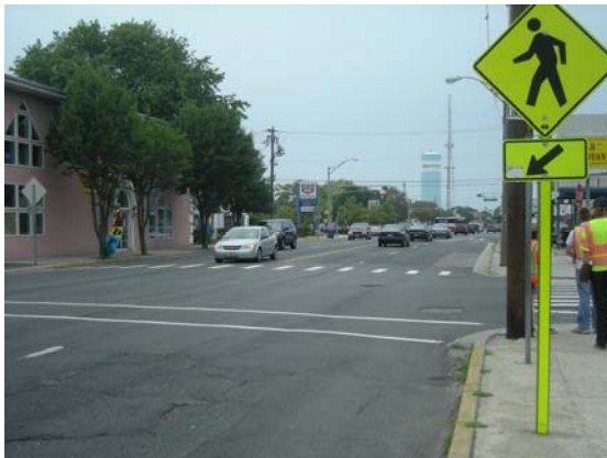
PICTURE 1: NO CURB RAMP AT CROSSWALK AT HEATHER ROAD
